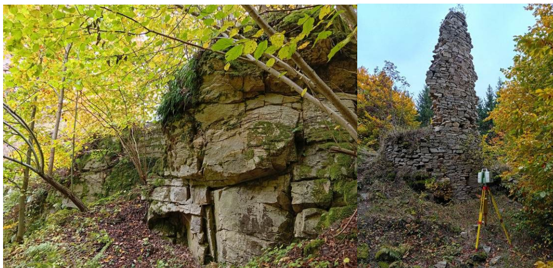
Fig. 2: Frost cliffs affected by weathering (left), Janštějn castle ruins (right). Photo: authors.
