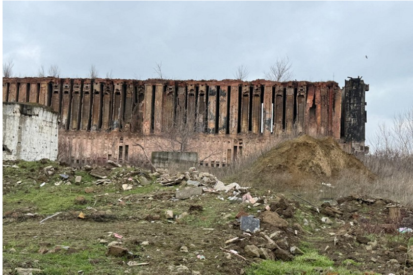
Fig. 1: The ruins of the power battery of the steel plant in Călărași
