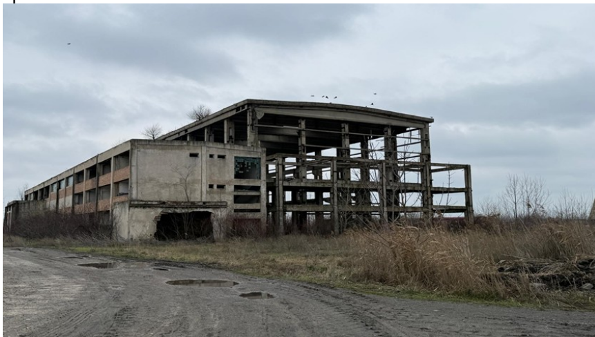
Fig. 3: The ruins of a drawbridge at the water cooling plant at the Călărași Steel Plant.
